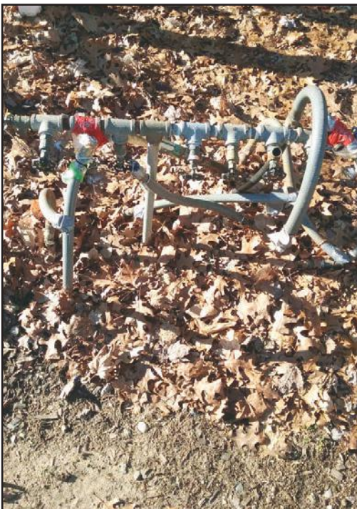
Old Water Riser
