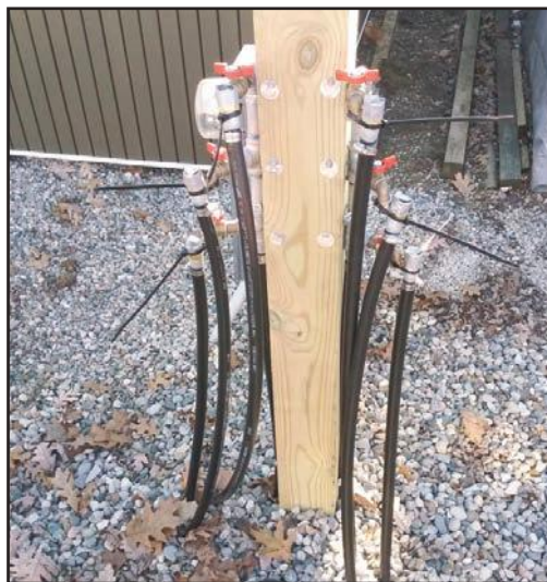
New Water Riser
